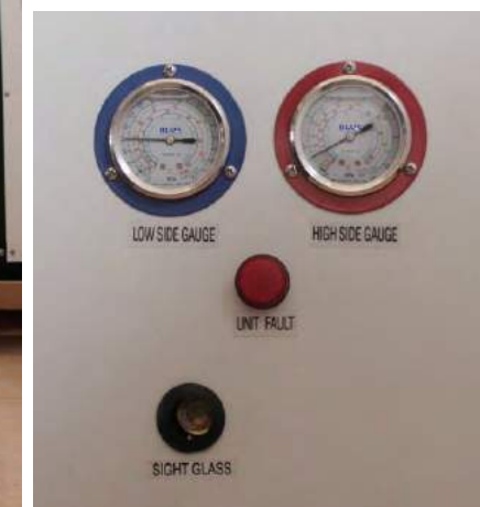
LP/HP Gauge Fault Warning Sight Glass
